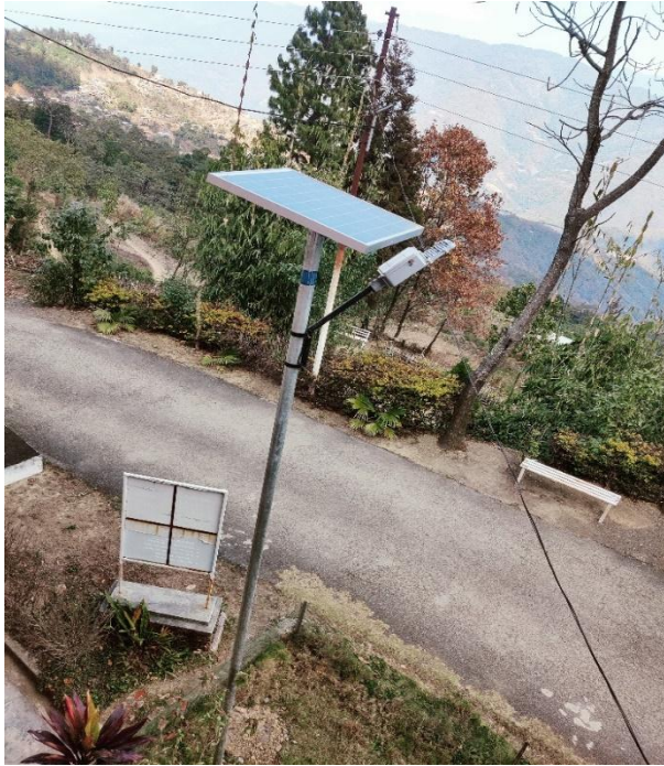
Figure 1: Picture of Solar Street light with sensor installed inside the campus
